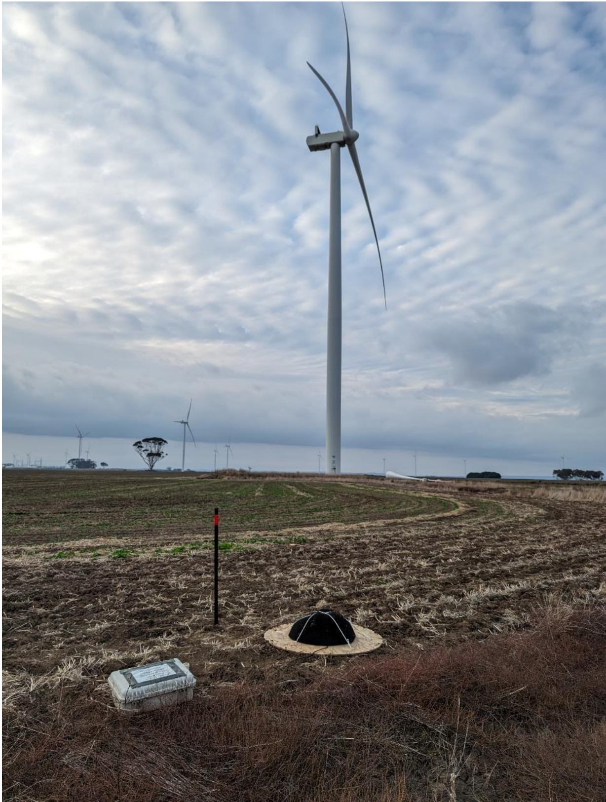
Figure 3: WTG.19 Primary Nearfield Monitoring Equipment
