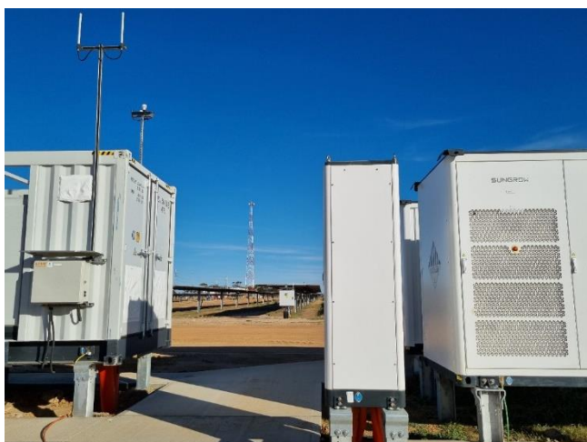
From this view, we can appreciate a battery, some solar panels and the communication tower
